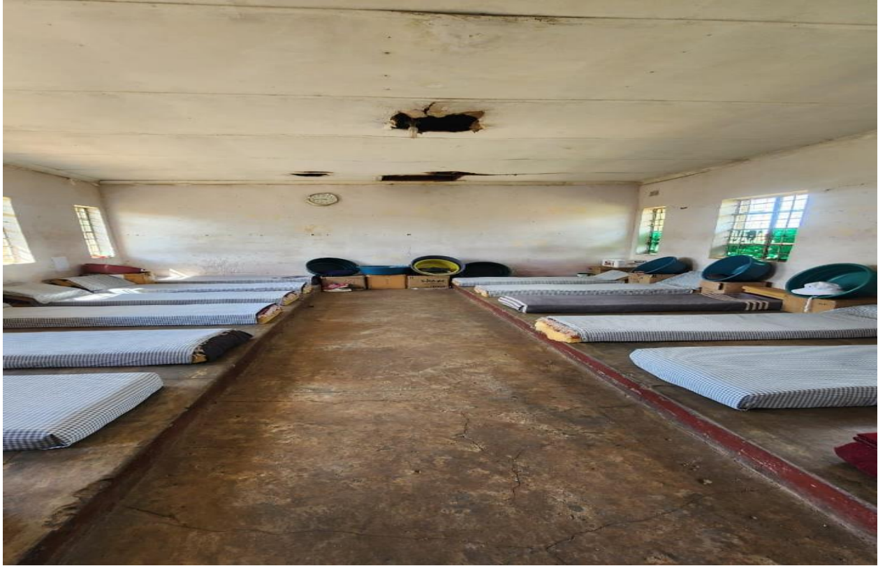
Fig 3: Maseru Female Correctional Facility Girls Dormitory ceilings
