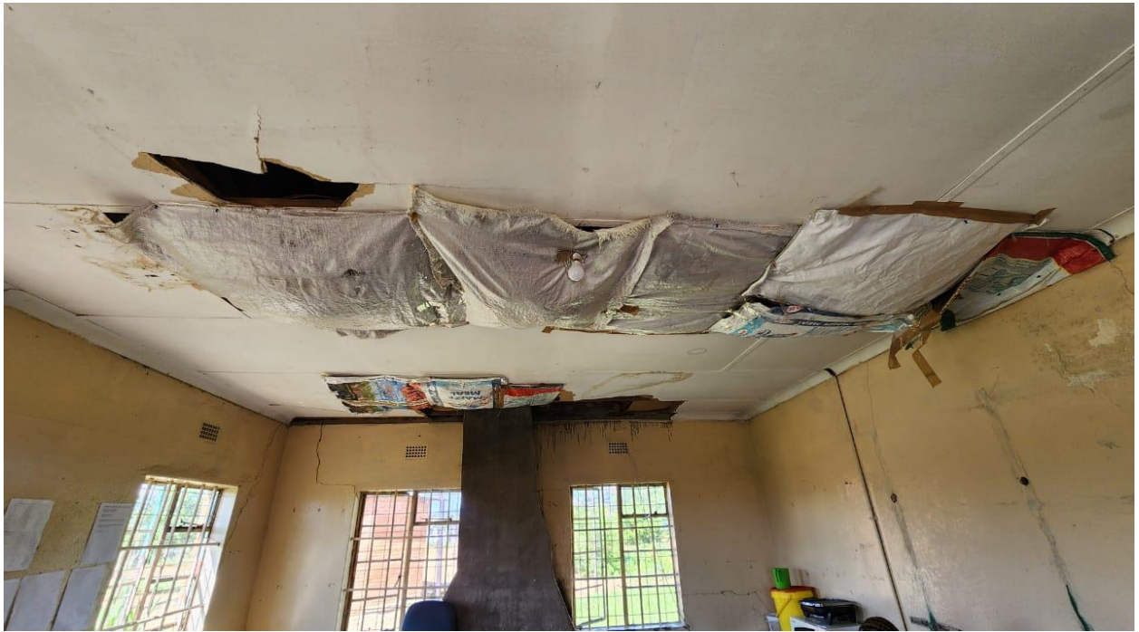
Fig 4: JTC Officer's Office ceilings
