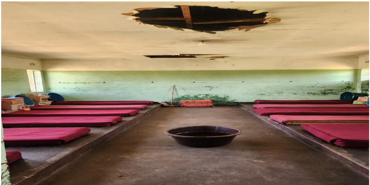
Fig 2: Maseru Female Correctional Facility ceilings
