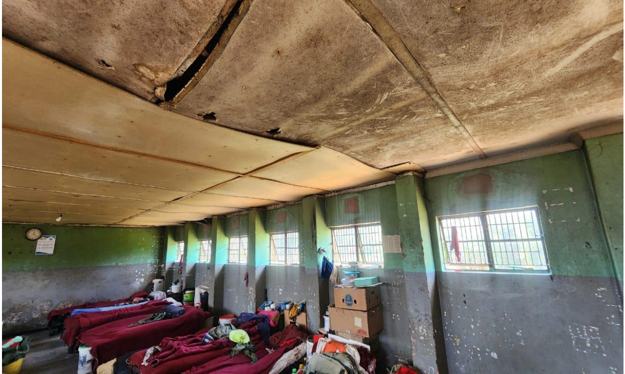
Figure 7: Lepereng Correctional Facility Ceilings
