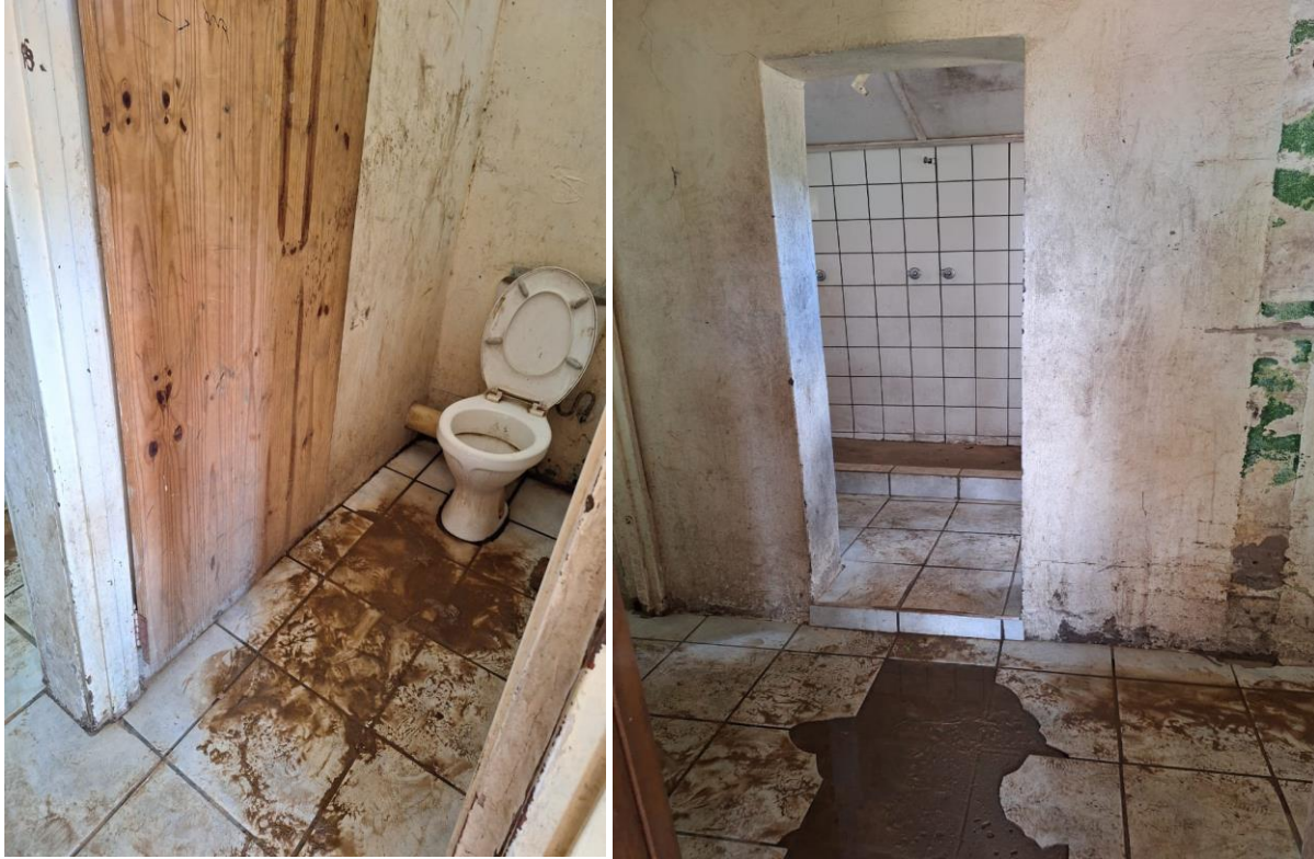
Figure 8 and figure 9: Dirty toilets and broken taps in shower
