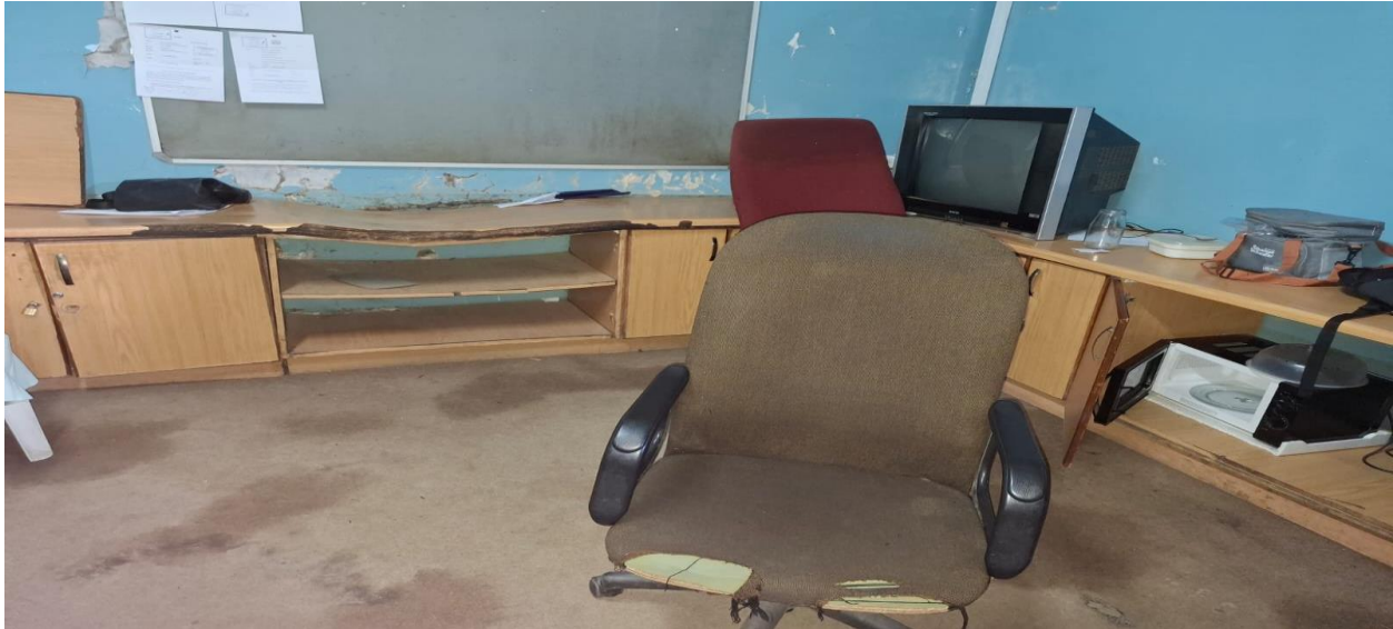
Figure 11: Broken furniture and equipment in LCS officers' office
