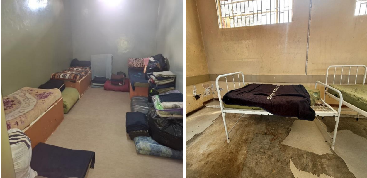
Figure 3 and figure 4: Mattresses and broken beds in forensic and male ward
