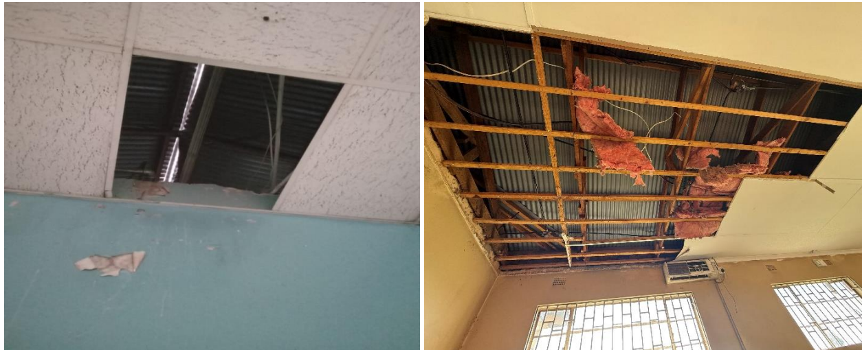
Figure 1: Dilapidated ceilings within the male ward and forensic unit
