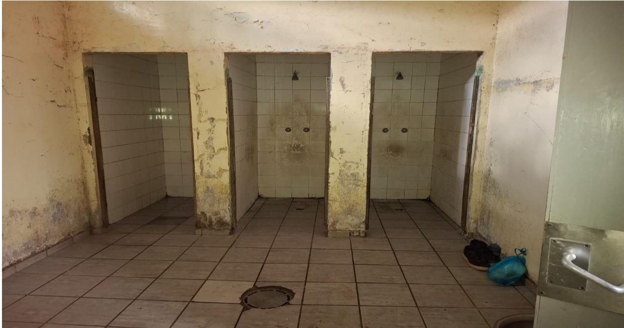
Figure 7: Showers without doors lacking privacy
