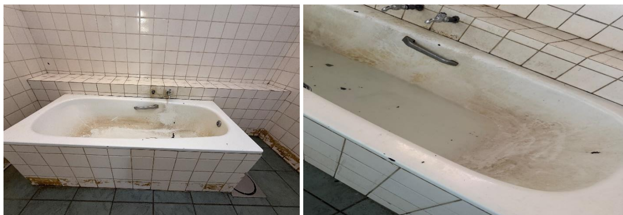
Figure 5 and figure 6: Blocked and unclean bathtubs
